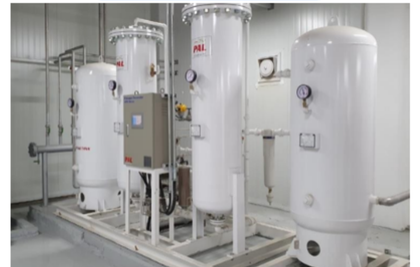
CO2 REMOVAL DRYER
